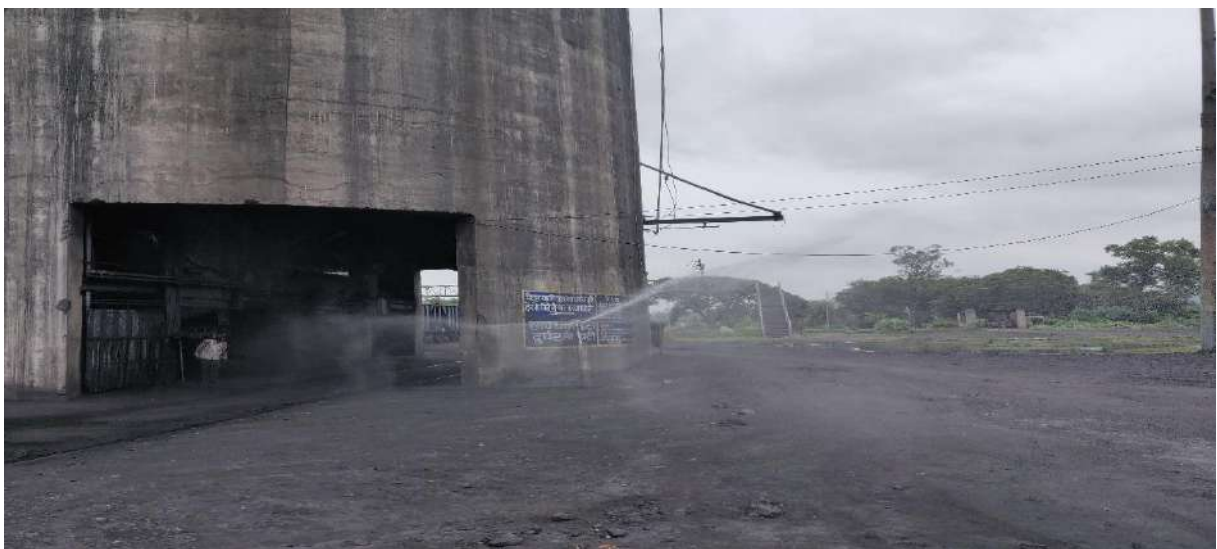
Photograph-3(c): Rotating fixed water sprinkler installed near silo dispatch
