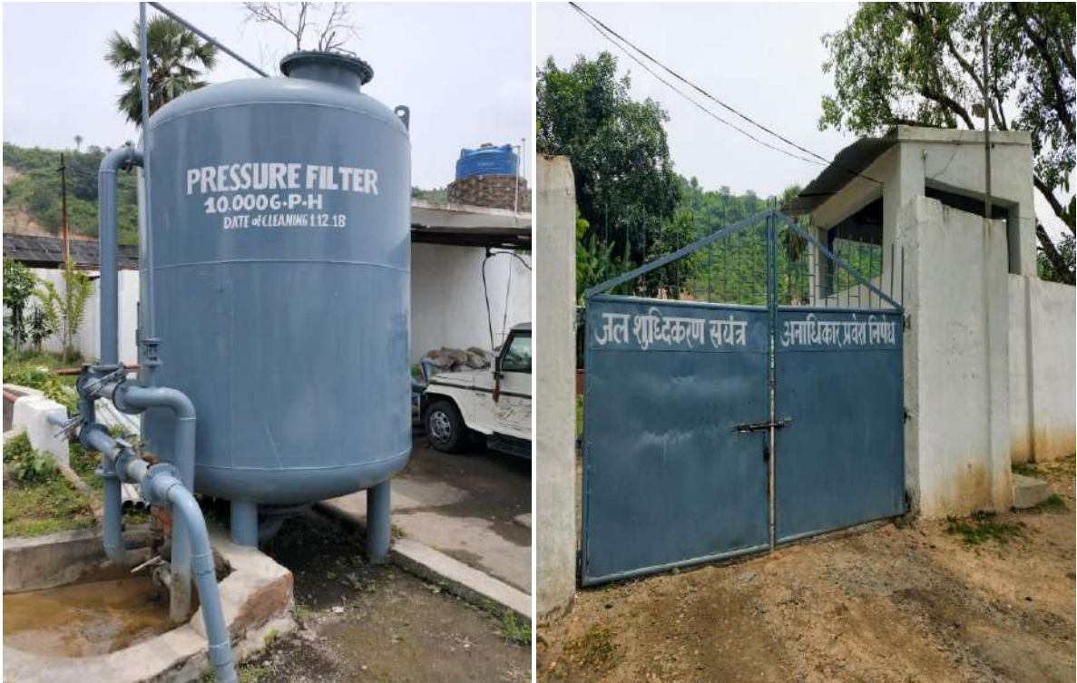
Photograph-5(a) , 5(b) : Lalmatia filtration plant
