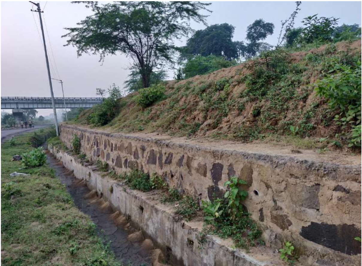
Photograph-4(b) : Toe walls and catch drains
