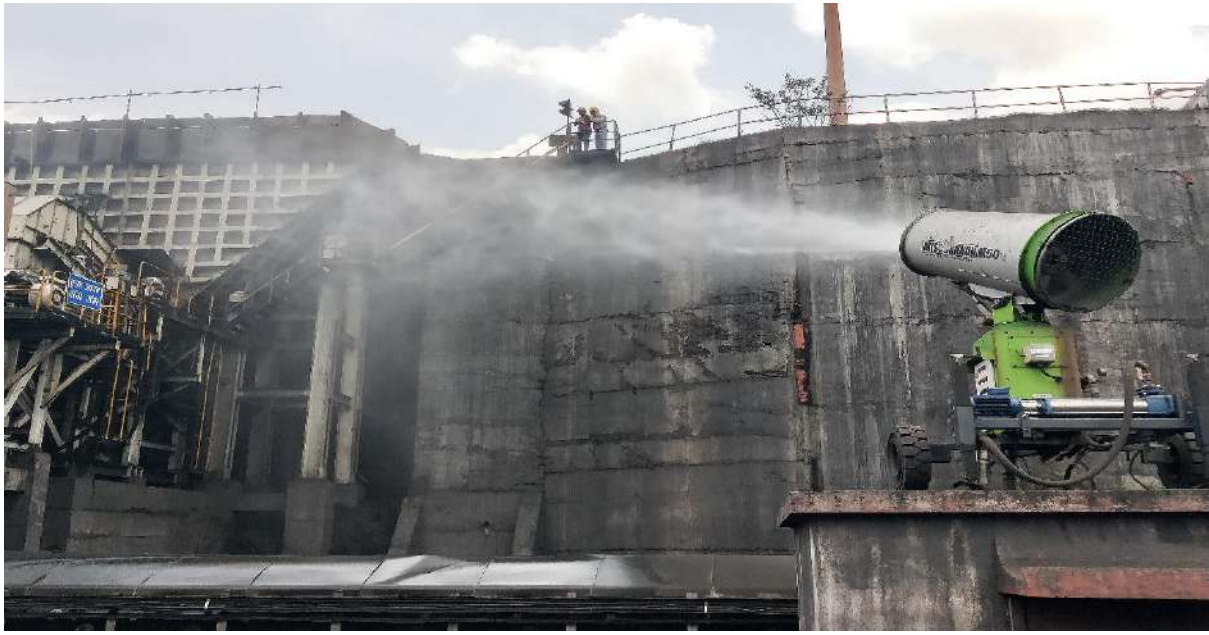
Photograph-3(a) Mist cannon installed near crushing point
